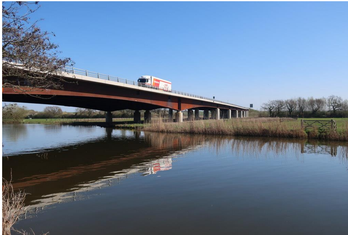
Figure 4 : Great Ouse Viaduct showing haunched soffit weathering steel beams contrasting with the concrete composite deck
